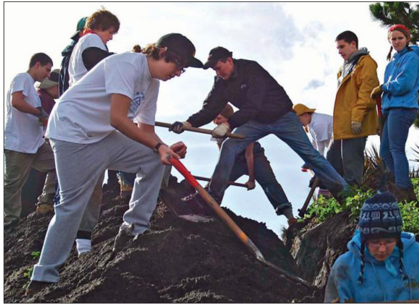
High school students from the Builders Beyond Borders program help install pipes that will carry water to the mountain town.
